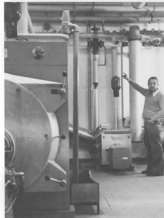
Erik Thoms, facilities engineering manager at HPSA in Geneva, shows how the large boiler on the left was replaced by the small unit and heat exchanger in the background, using 95 percent less fuel to do the same job. Phenomenal savings have been realized by recovering heat from the building’s computers and improving the flow and regulation of air-conditioning, according to Erik, and solar heat is used for domestic hot water. At Swiss fuel prices, the cost of transforming HP’s European headquarters into an energy-efficient building has paid for itself in three years.
